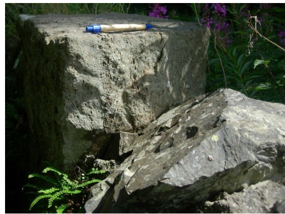
Fig. 8 – Vertical-bedded sandstone in the wall.
