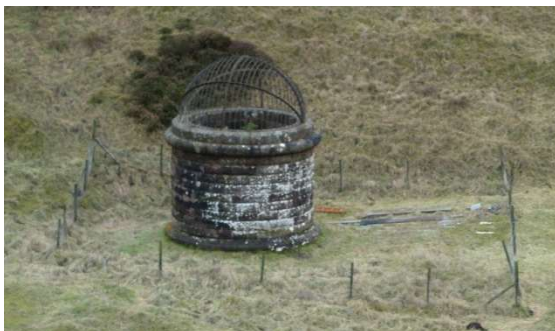
Fig 7: Ventilation shaft cover for the Talla Aqueduct
